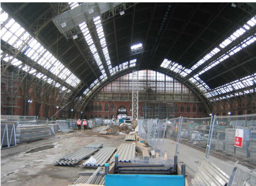
New train shed being built at St. Pancras Station, London, the final terminus for Eurostar service to Paris. — Photo by Michael Kiesling
